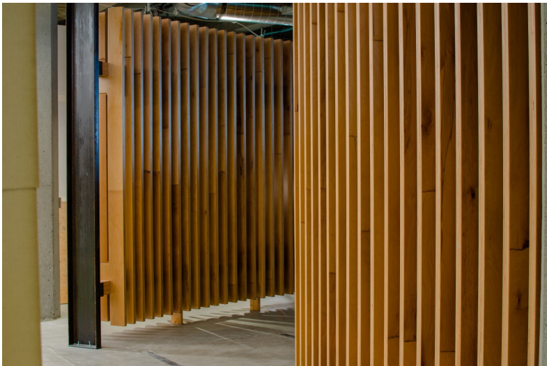
Photos of a local distribution giant in downtown Seattle, WA. 9 floors of industrial-looking Doug Fir. All provided by AWI/QCP Member Interior Woodworking Specialists (I.W.S.)
